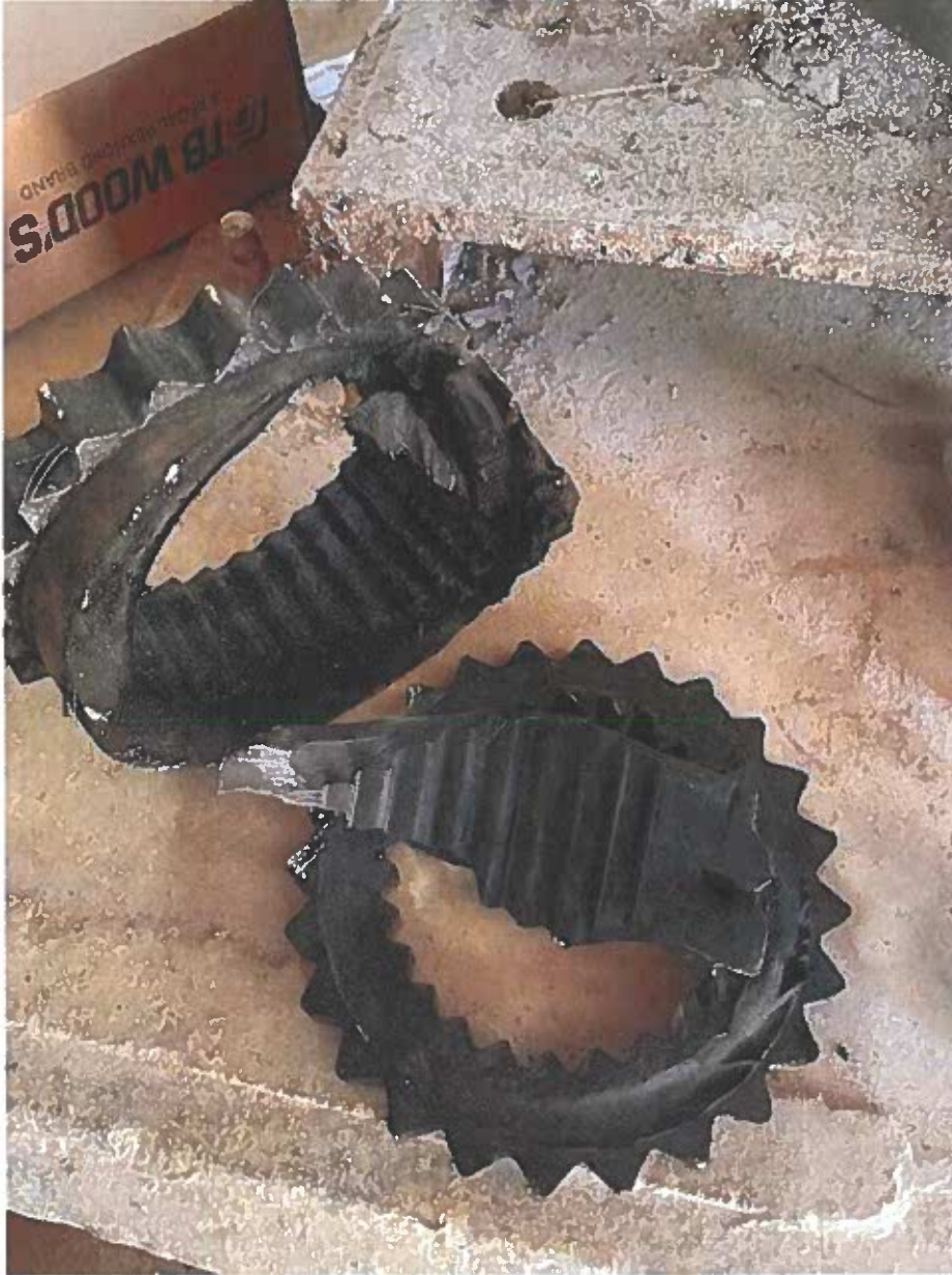
Photo #1 - HS Pump #2 Coupler
