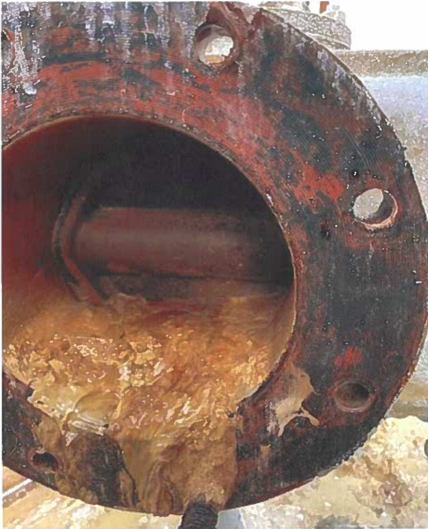
Photo #4 - Lime Buildup in Low Service Pump Effluent Line
