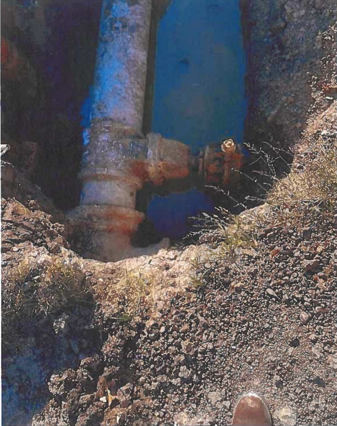
Photo #3 - High Service Pump Station Valve
