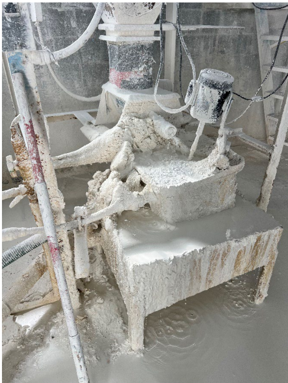
Figure 27: Lime Mixer Basin for Clarifier #2
