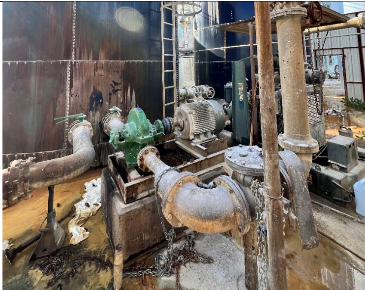
Figure 19: Low Service Pump Station
