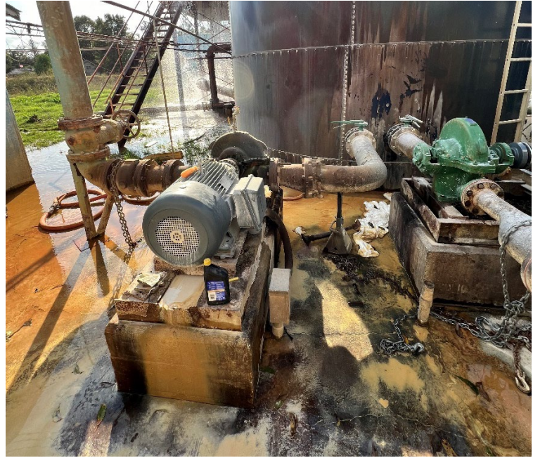
Figure 18: Low Service Pump Station
