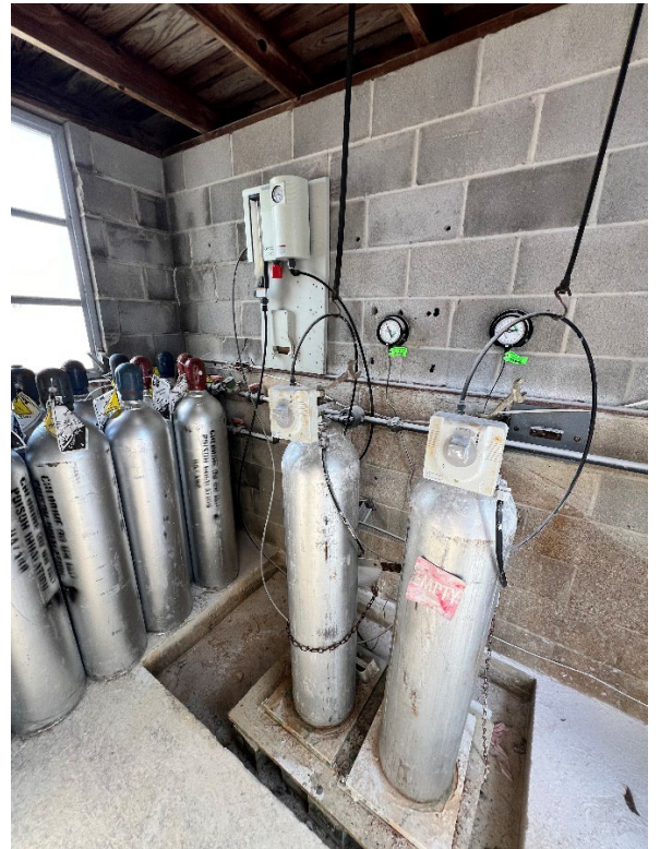
Figure 30: Chlorine Feed System
