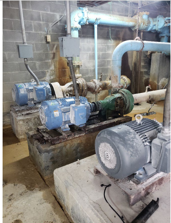
Figure 24: High Service Pumps
