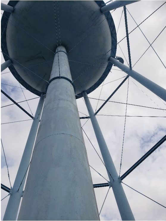
Figure 23: Elevated Storage Tank
