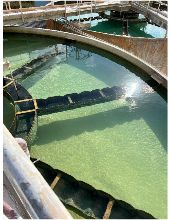
Figure 10: Solids Contact Clarifier #1
