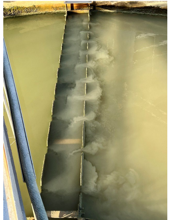
Figure 12: Solids Contact Clarifier #1 Launderers
