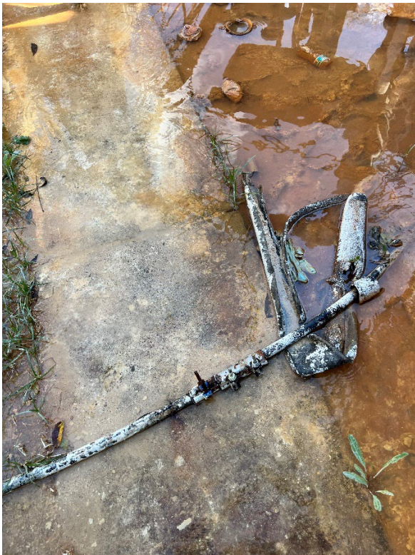
Figure 31: Chlorine Feed Line Underwater
